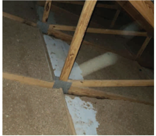
Uninsulated area in attic caused by settled insulation. Photo Credit: Insul-Pro Plus
