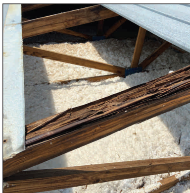
Rotten trusses from fastener leaks
